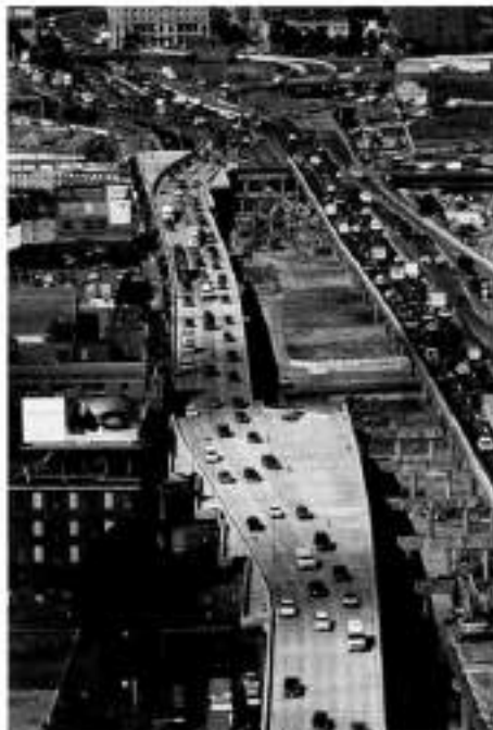
PHOTO COURTESY OF BOSTON CENTRAL ARTERIAL/TUNNEL PROJECT Traffic continues to flow as construction proceeds on Big Dig.
