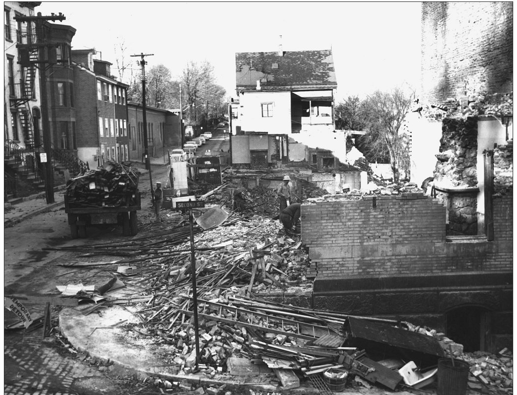
During urban renewal in Newburgh, New York, an old firehouse on the corner of Second and Montgomery Streets was demolished. Courtesy of Historical Society of Newburgh.
