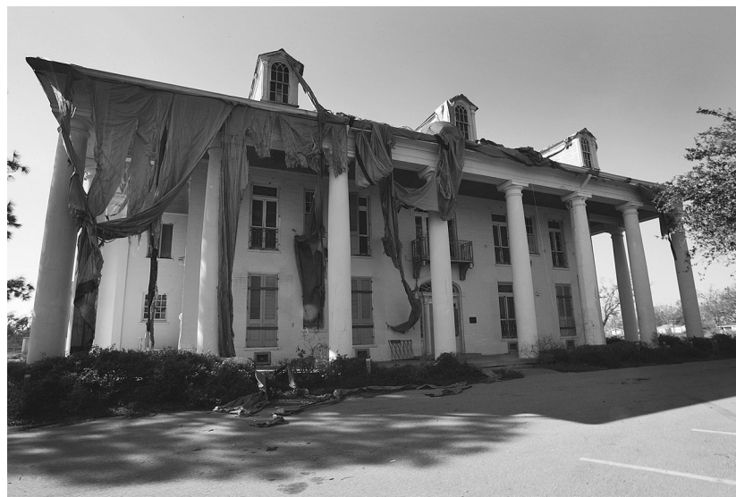
Shredded blue tarps, used as emergency roof repairs, hang from the roof of the Milne Boys Home in New Orleans. January 26, 2007.
