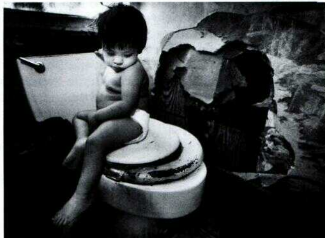
Roberto Flores sits in an Apopka, Florida, apartment that the landlord refuses to fix. "The sewage leaks into the kitchen when it rains," says his mother, Maria Santana. "And the baby gets rashes all over his body." They have since moved.
