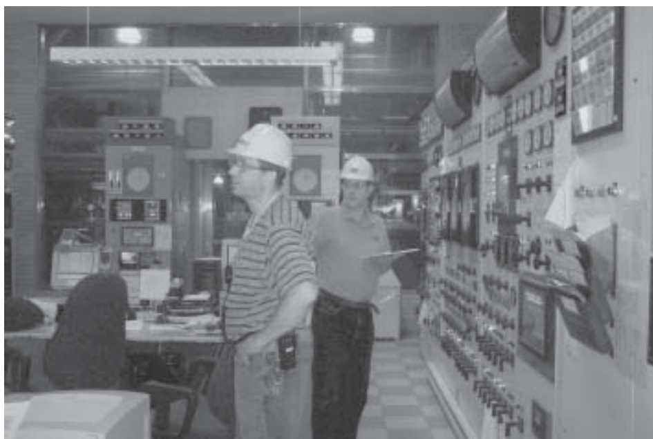
Wayne Bolton-Engelhardt and a colleague in the control room at the Albany Steam Station. Photo by Mark Clayton.
