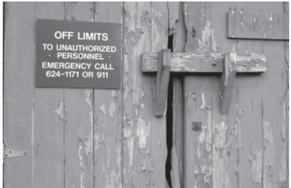
The paint peels off the wood of a World War II-era barrack where soldiers on medical hold were originally placed on their arrival at Fort Knox in Kentucky. These soldiers were later moved to what the Army says are better living conditions. One of the barrack’s roofs collapsed two days after soldiers were moved out. Photo by Michael Kleinfeld/UPI.
