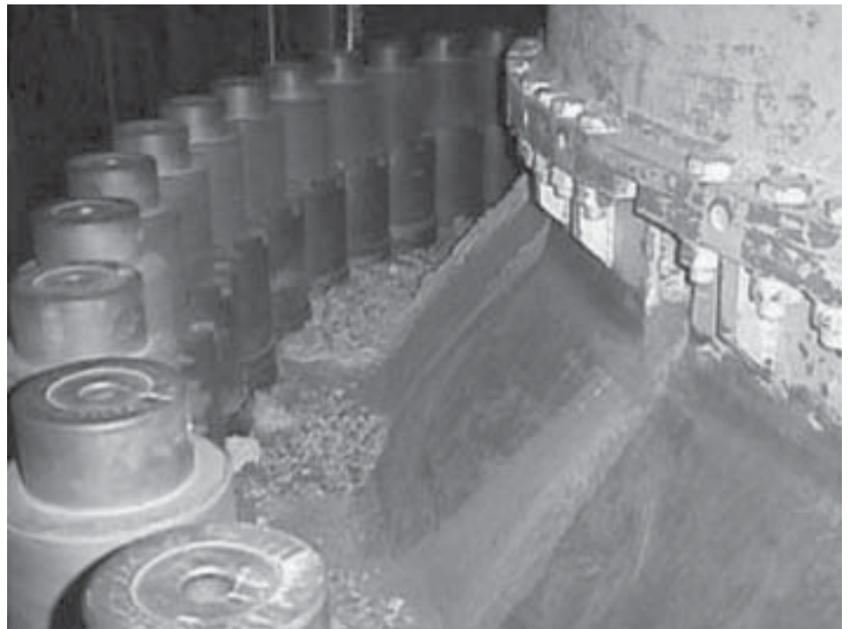
This photo of the lid of the Davis-Besse reactor was taken during a refueling in April 2000. It shows where rust and dried boric acid were streaming off the reactor's lid nearly two years before the rust hole was detected. This was one of a set of photos handed by workers to an inspector for the Nuclear Regulatory Commission in 2000—but never acted on. Photo by David I. Andersen/The Plain Dealer.
